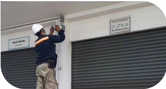
Wireless CCTV and Fire Alarm systems.
