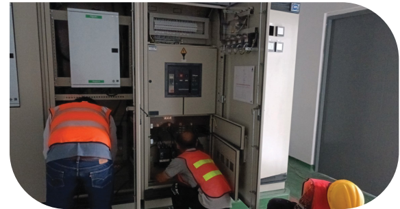
Control Systems and energy-saving systems.
